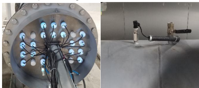
Water treatment systems operating examples
