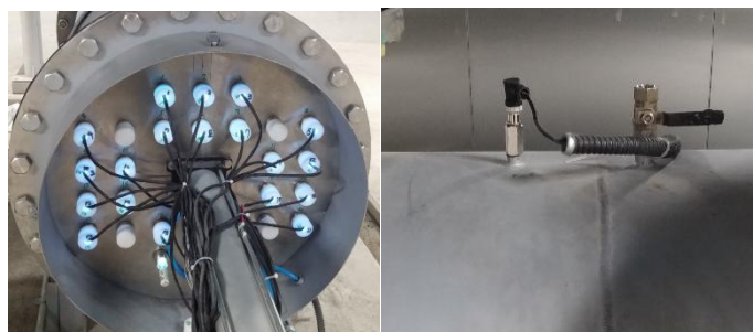
Water treatment systems operating examples
